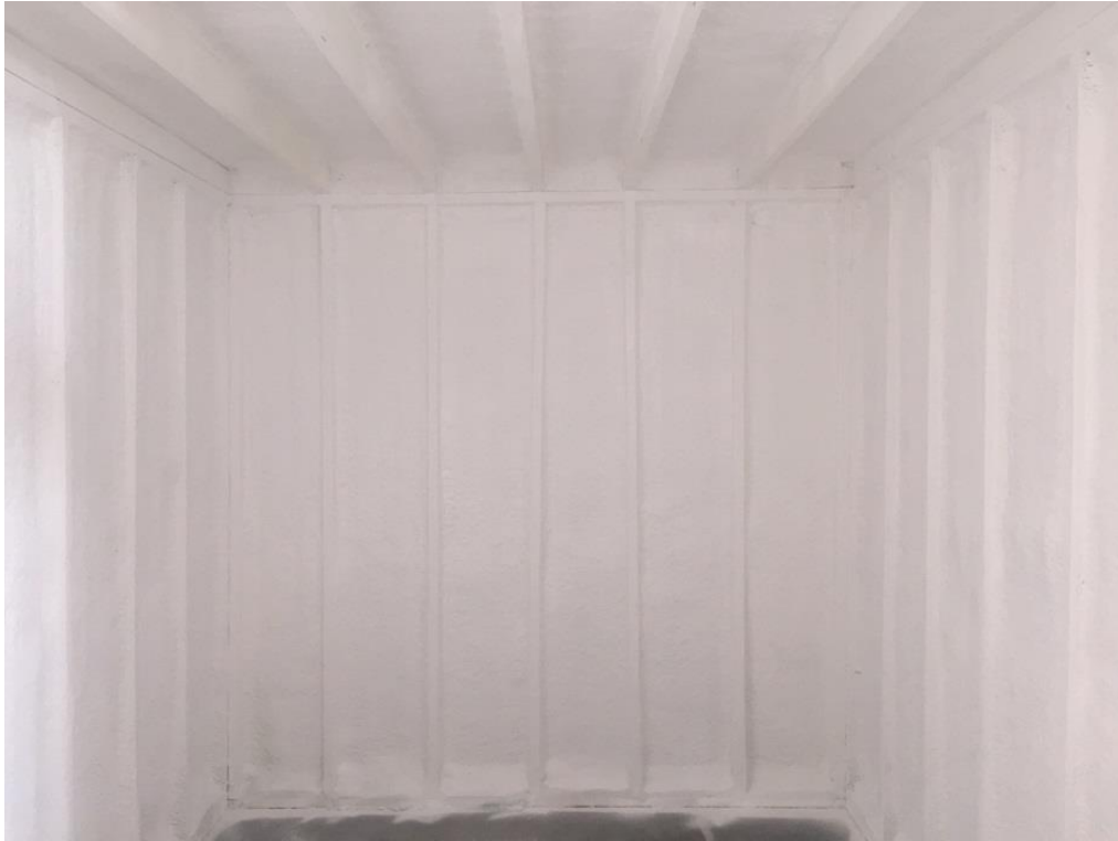
Figure 2. Example of application where DC 315 (white) serves as the thermal barrier over MD spray urethane cavity insulation (and overexposed studs/joists) 1 in wood-frame basement walls and ceiling.
